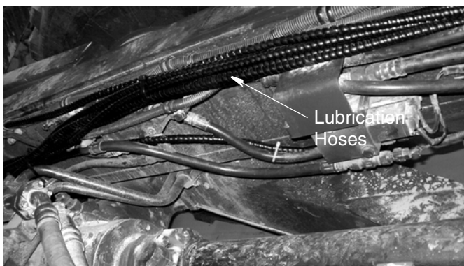
FIG. 108: Hoses running along left side dump body frame rail to back of truck dump bed on HM300-5.
